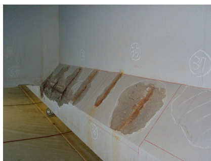
Phot.2 Deterioration after repair
