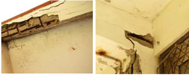
Figure 1. Corroded members of reinforced concrete buildings
