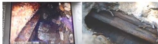
Photo.2 Corrosion of PC cable
