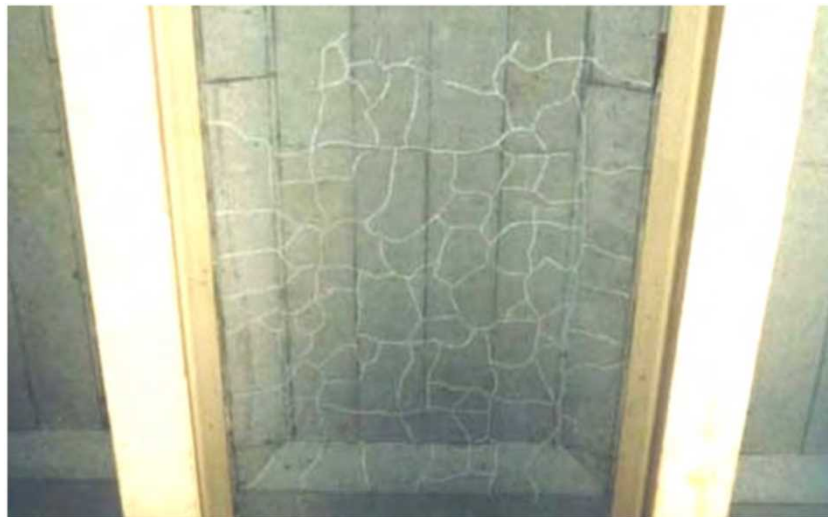
Bottom surface of a fatigue damaged RC bridge deck
