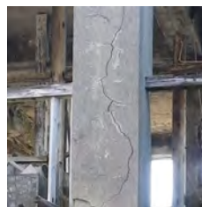
B) Concrete cracked or detached due to rebar corrosion
