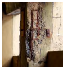
C) Cover concrete spalled off and rebars exposed
